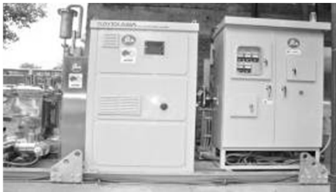
EHP installed in Milkfed (June 2013)
