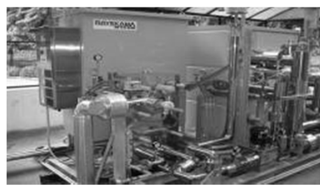
EHP installed in Amul (July 2013)
